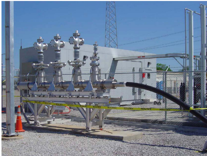
200 meters, 13.2 kV, 3kA, American Electric Power, Columbus, OH, in service Sept 06
